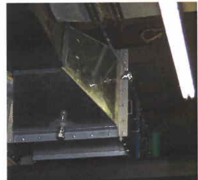
Delaware Valley's First Heat Exchanger
